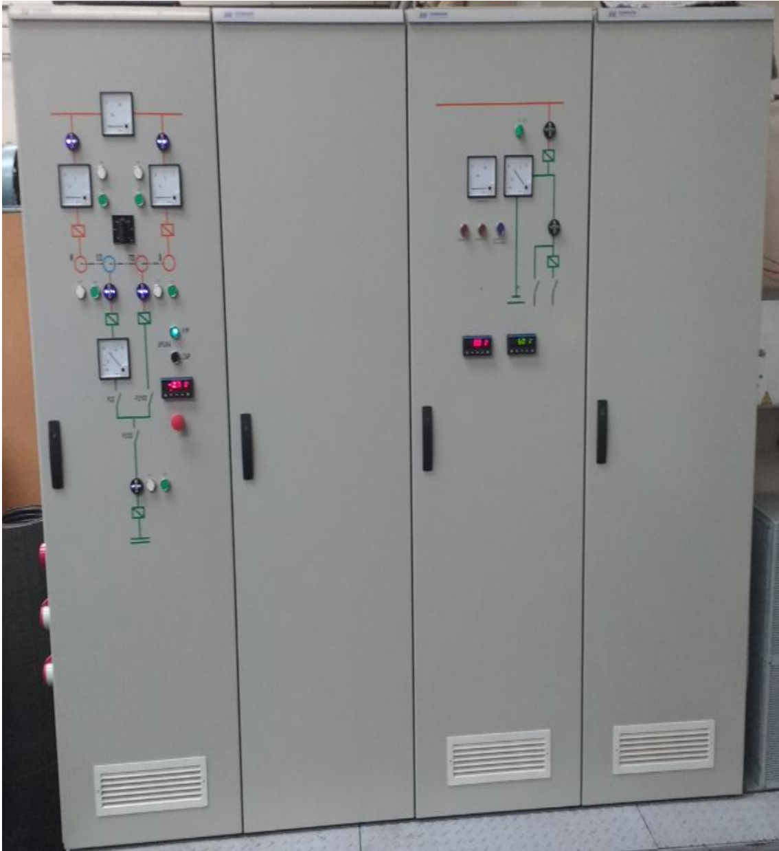
Figure 6.6: Other necessary equipment in this control chamber.
